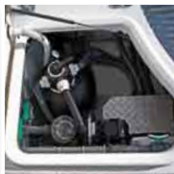
All the equipment is pre-installed in the technique shaft under the shower tray.
